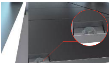
Car battery swap station chassis positioning detection
